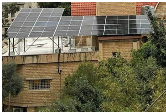
Solar panels provide a consistent power source despite the frequent blackouts and high fuel costs affecting Lebanon.
